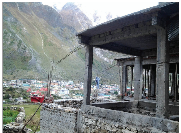
North east corner: pillars for office/bookstore in foreground, and meditation hall behind.
